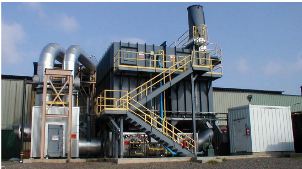
Regenerative catalytic oxidizer on a veneer dryer at Weyerhaeuser plant in Zwolle, La.
