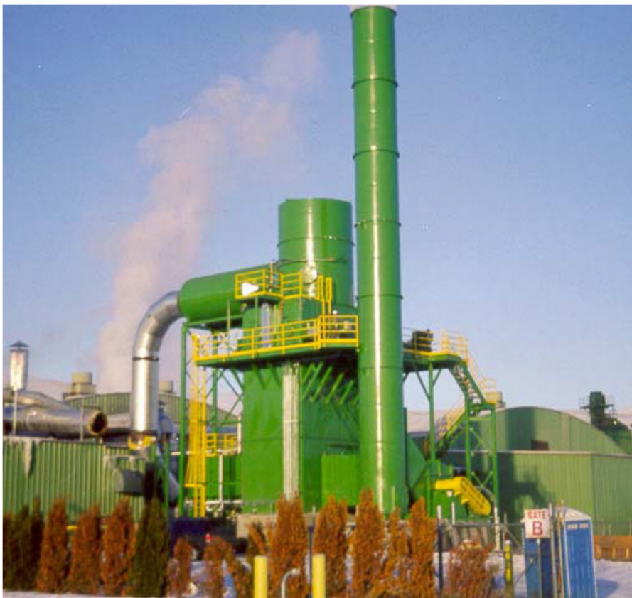
Wet ESP on a plywood veneer dryer at Boise in Yakima, Wash.
